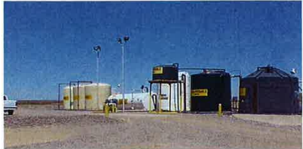
Photo 3: Solution storage tanks at the Florence Copper Project site
