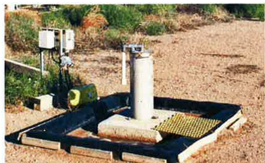
Photo 4: An injection well at the Florence Copper Project site
